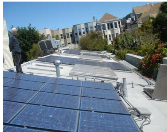
Rosebud's 10-kW solar PV system supplies 100% of its electricity needs
