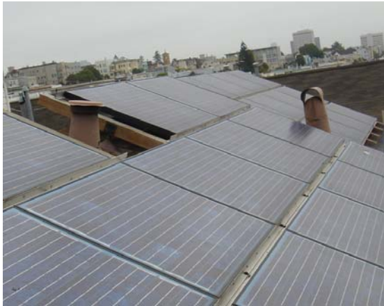
Yoga Garden's 3-kW solar array.
