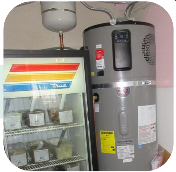
Figure 1: Hybrid heat pump in a small establishment
