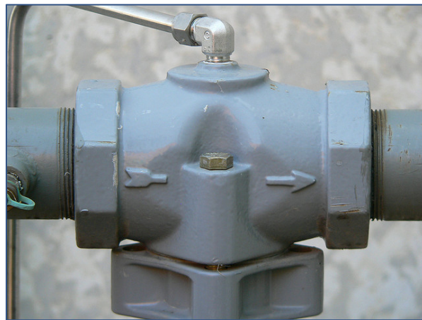
Natural gas pipeline outside of a building Photo Credit: Flickr Creative Commons / ericeggertson
